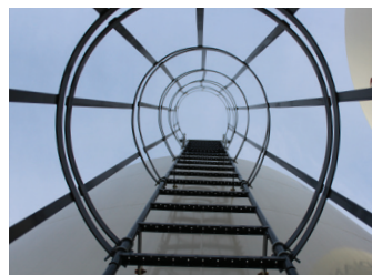
Ladder Cage & Handrails
