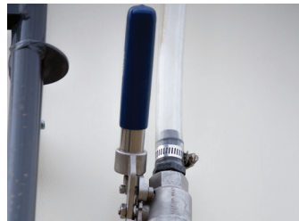
Liquid Site Gauge Valve
